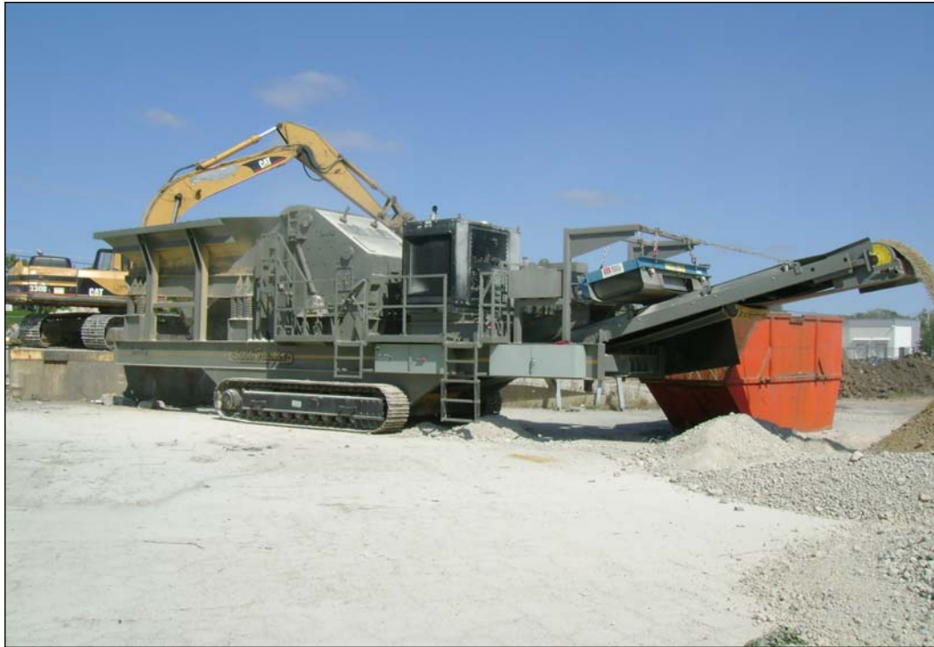
Inertia Machine’s 5066 Tracker features Rulmecca Motorized Pulley model 400M at 15 HP to move up to 700 tph of crushed product on 42” belt at 300 fpm, using 460v/3ph/60Hz power supply.
